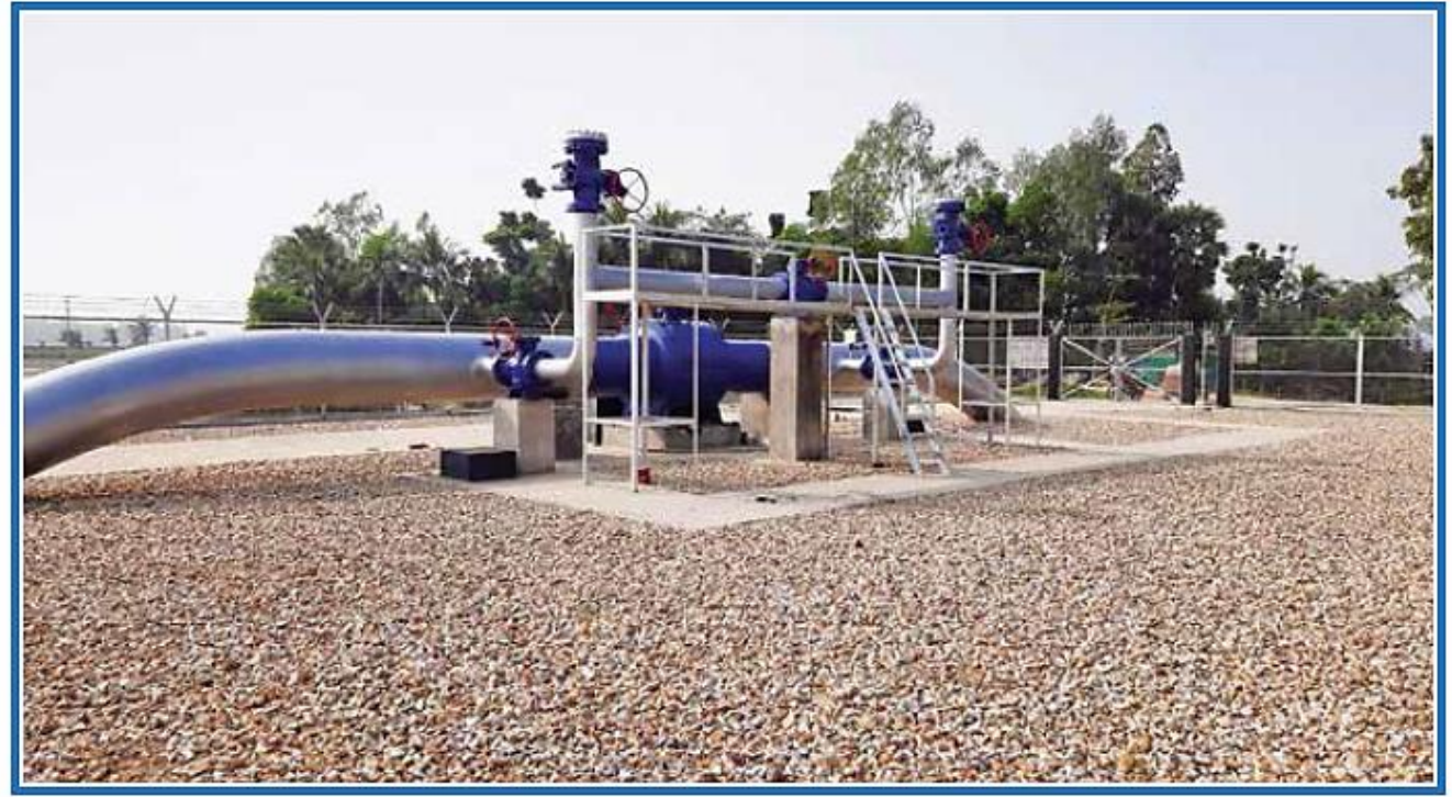
Valve Station Under Chattogram-Feni-Bakhrabad project
