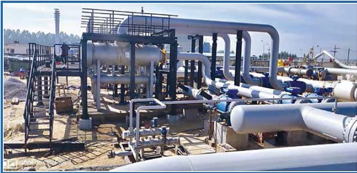
1500 million cubic feet capacity metering station constructing under Maheshkhali Zero point project
